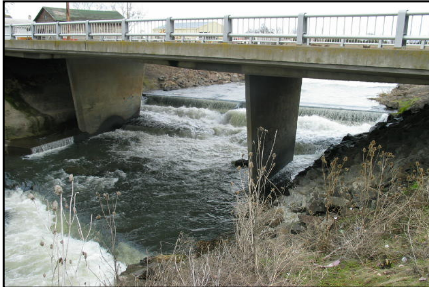
Figure 13: This pre-project photo was taken in 2004. In this condition, migrating salmonid fish were unable to negotiate the series of structures under most flow conditions.
