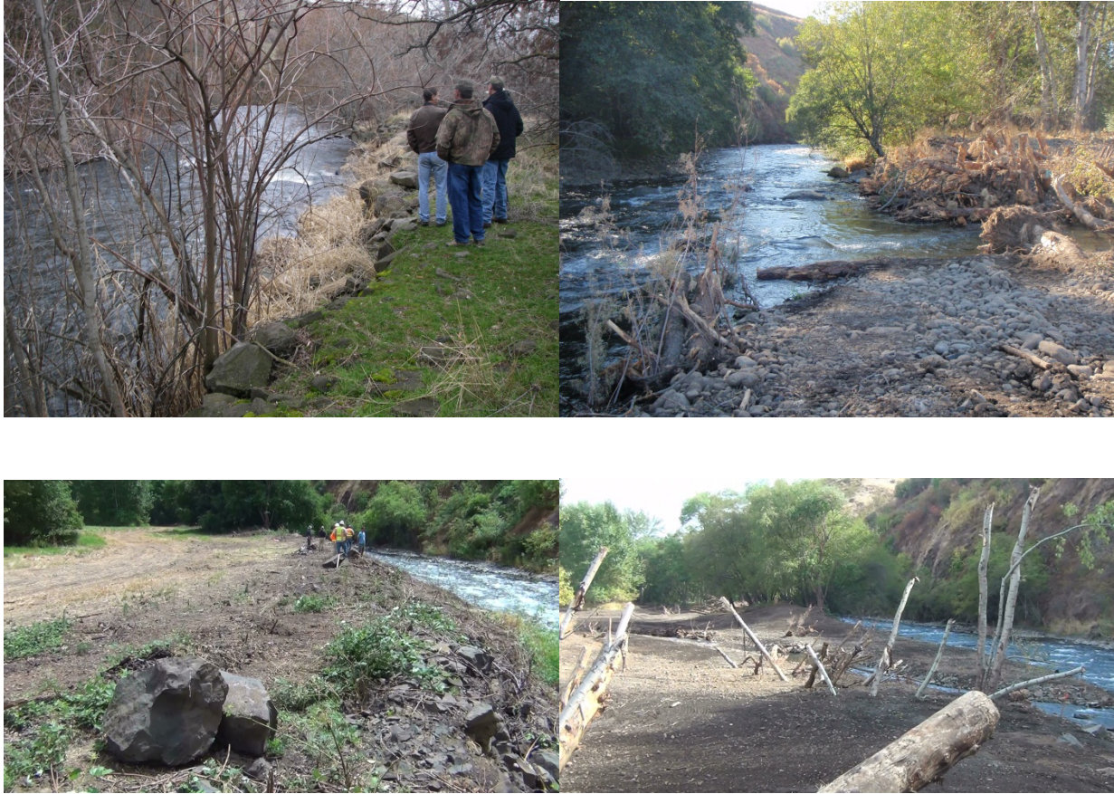
Figure 6: A series of before (on the left) and after (on the right) photos of the construction site. The side channel entrance is shown in the center photo on the right.
