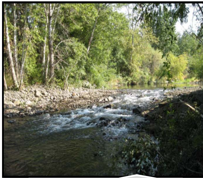
Photo looking upstream at the completed project site. The roughened channel was constructed to maintain a slope that fish can negotiate
