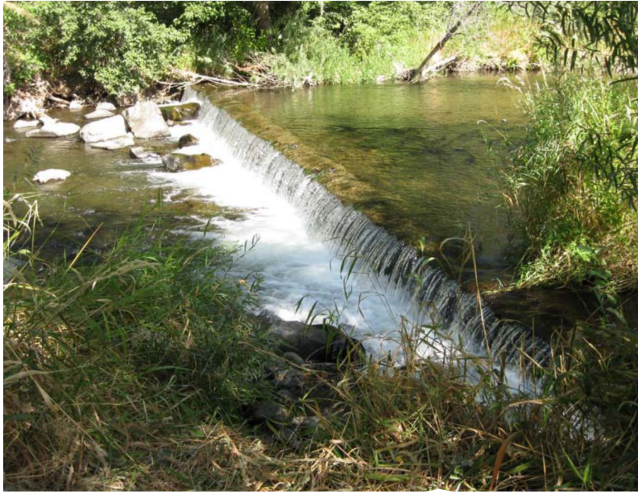
This pre construction photo shows the fish passage barrier. The structure was originally built in the 1940s
