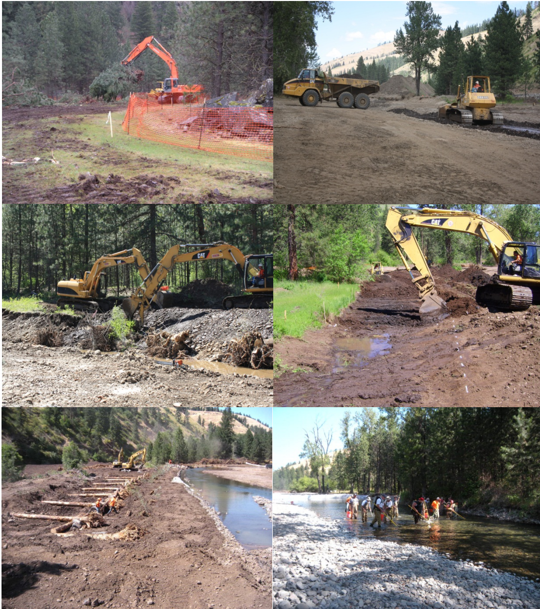
Figure 15. Implementation photos of the Meacham Creek Floodplain Restoration and In-stream Enhancement Project RM 6-7.1; photos from top right going clockwise: 1-installing stream bed gravel, 2-excavating new channel, 3-fish salvage, 4-installation of diversion plug, 5-installing habitat structures, and 6-clearing and grubbing project area.
