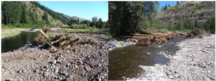
Photos of large woody debris constructed on the Meacham Creek Phase II RM 6-8.5 Project
