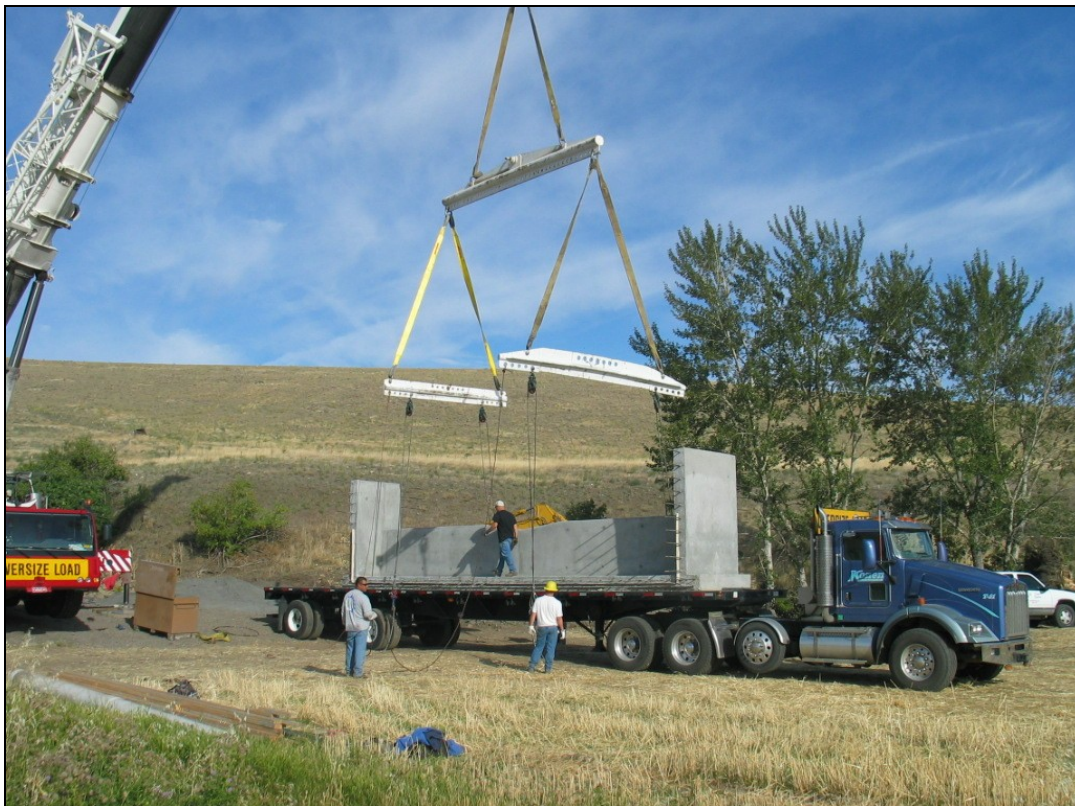
Figure 28. One of the Thirteen Sections of the Fishway
