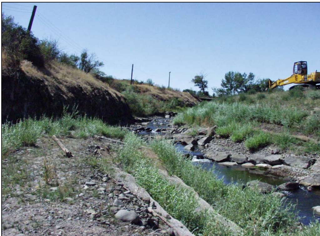
Figure 12. Weinke Dam Passage Rectification Project Partnership with ODFW Showing Progress of Willow Plantings, Birch Creek, RM 15.5 – July 2008
