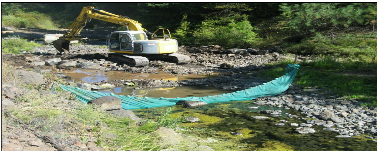
Figure 22. Meacham Creek RM 20.2 Construction of Upper Cross Vein Showing Site Isolation Method
