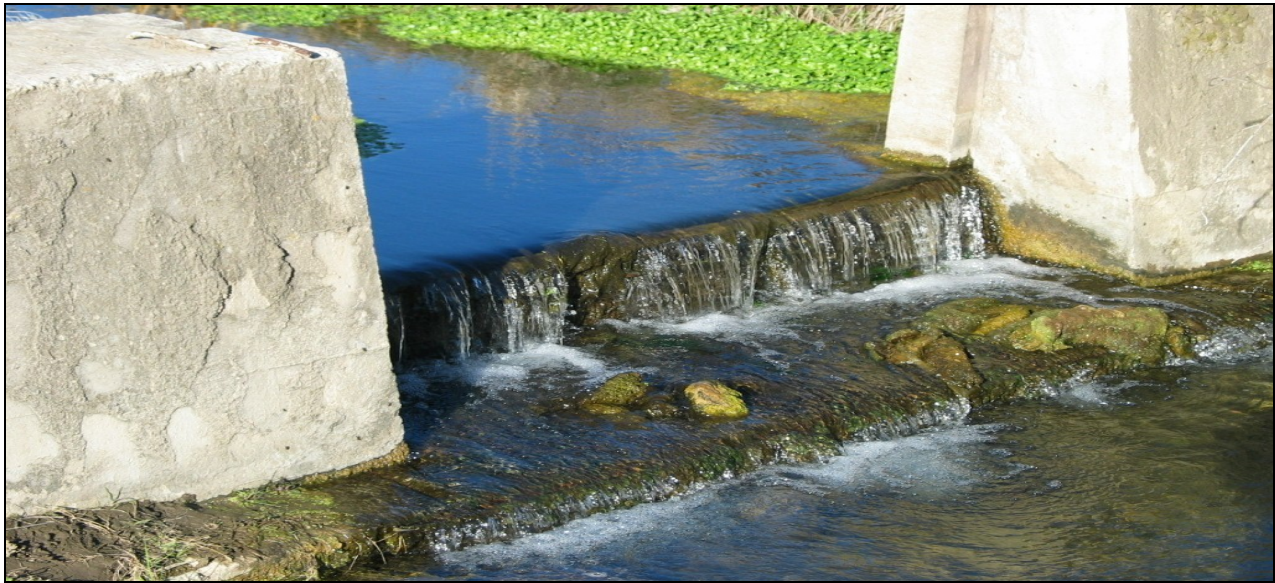
Figure 25. Greasewood Creek Fish Passage Barrier, RM 0.4 Prior to Rectification
