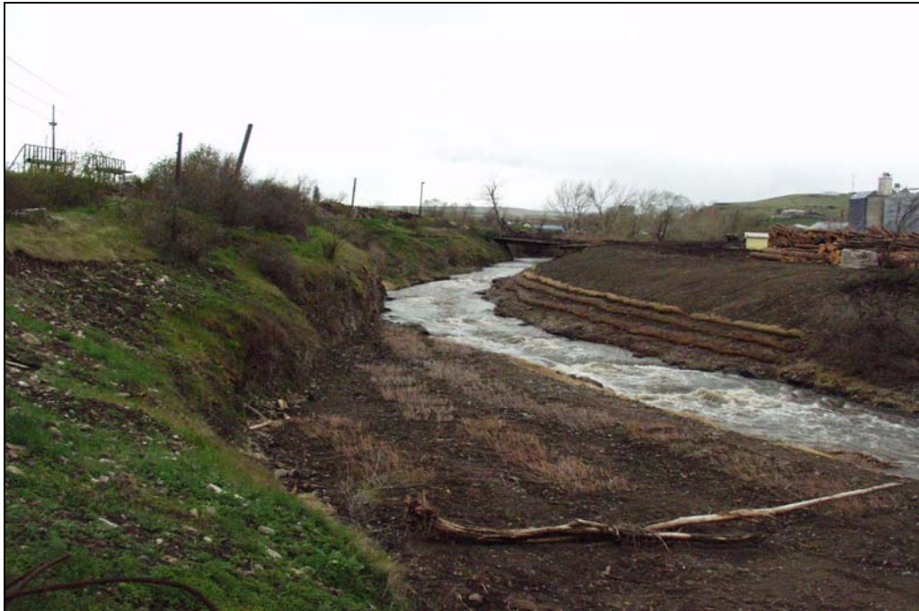
Figure 11. Weinke Dam Passage Rectification Project Partnership with ODFW Showing Willow Plantings, Birch Creek, RM 15.5 - December 2007
