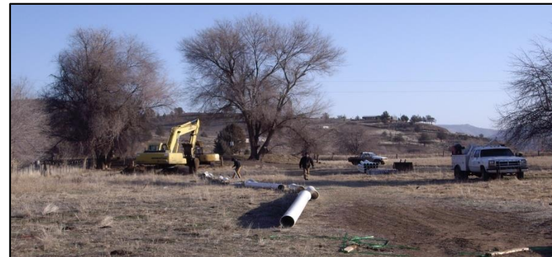
Preparing to bury water lines for the NFJD Push-up Dam Relocation Project
