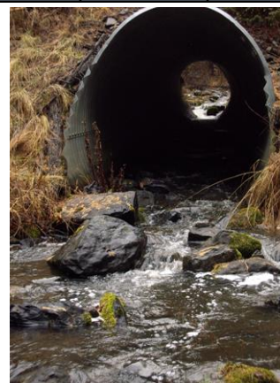
Undersized culvert on Battle Creek
