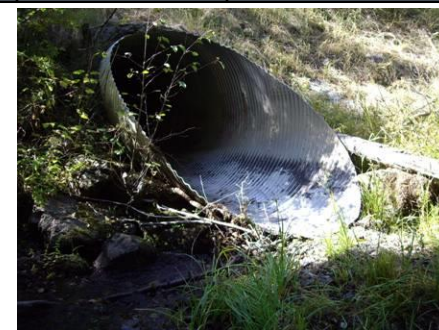
Undersized culvert on Bruin Creek
