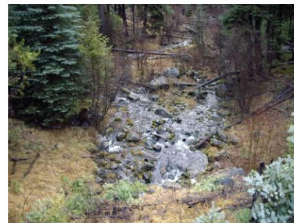
Battle Creek below undersized culvert
