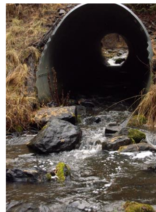
Undersized culvert on Battle Creek
