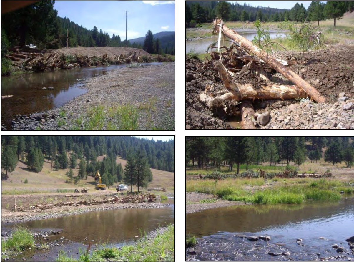
Figure 27. Structures placed along Granite Creek to reduce streambank erosion and increase channel complexity from upstream (top left) to downstream (bottom right).
