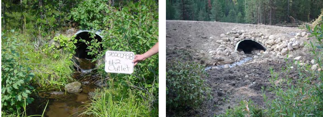
Figure 10. Original middle Ten Cent Creek culvert (left) replaced by a bottomless arch on footers in 2012.
