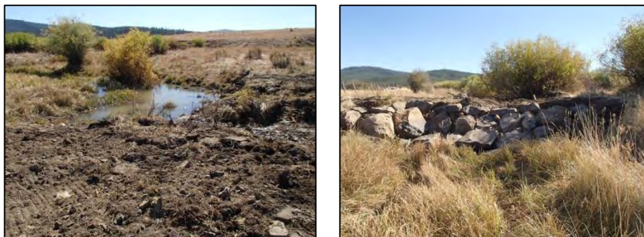
Figure 13. Pictures from after implementation showing water backed up above the plug (left) immediately after implementation and the plug from the downstream side (right).
