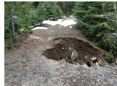
Little Indian Creek culvert failure.
