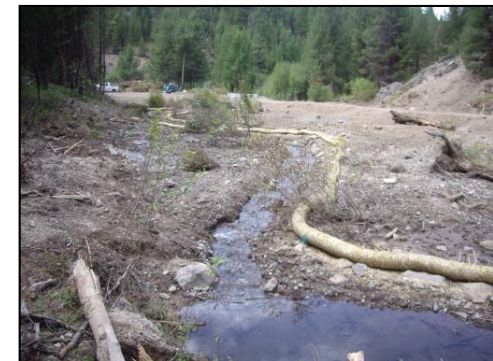
Right - Looking downstream at the new pre-cast concrete bridge across Deep Creek. The picture also shows the realigned and roughed out stream channel.
