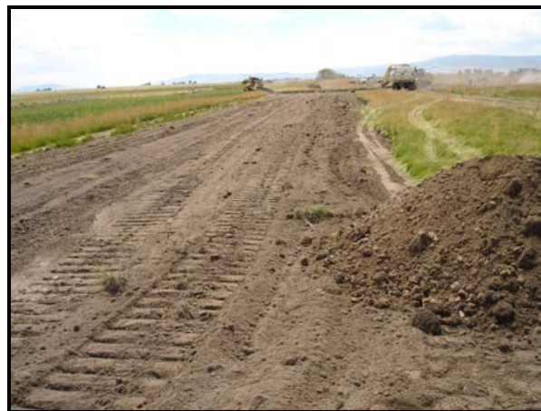
Earthen terrace constructed along eastern project boundary to minimize potential for flooding on adjacent private land. July 2006
