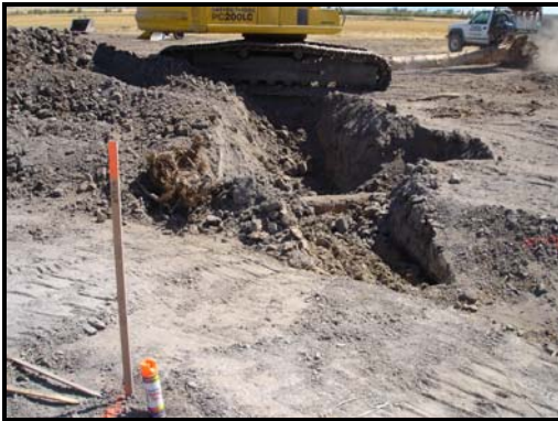
Rootwad revetment installation. Photo illustrates installed footer log and keyway for rootwad and tree bole installation. August 2006
