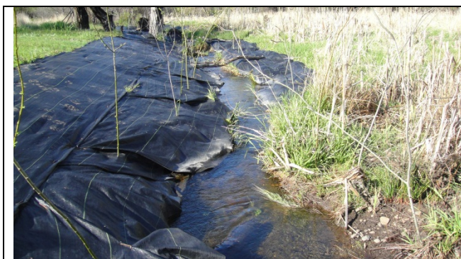
Actively Eroding Bank and High Terrace
