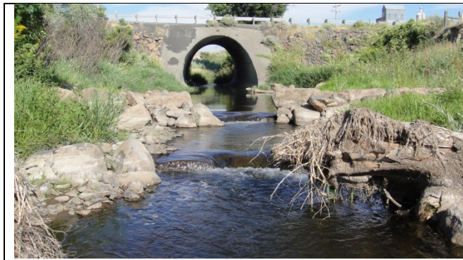
Actively Eroding Bank and High Terrace
