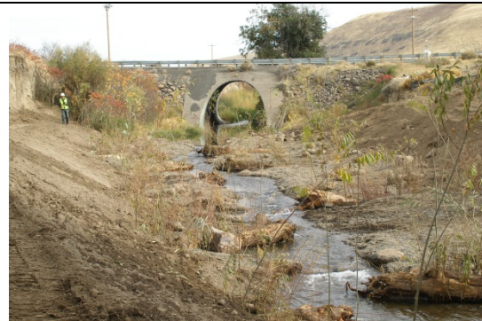
Large Wood Debris Accumulation
