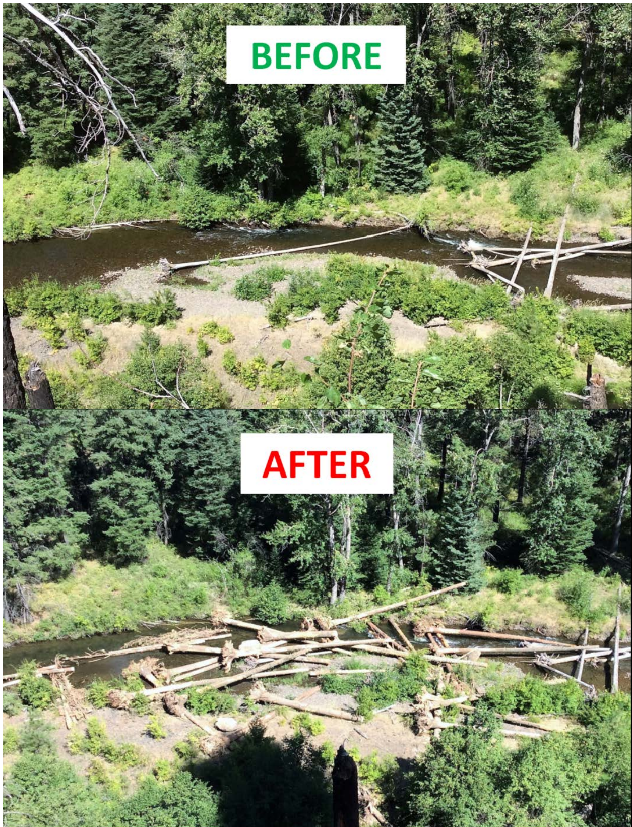
Figure 13: Pre-treatment and post-treatment conditions where a channel spanning wood structure was placed near the upstream opening to a paleochannel in PA3.
