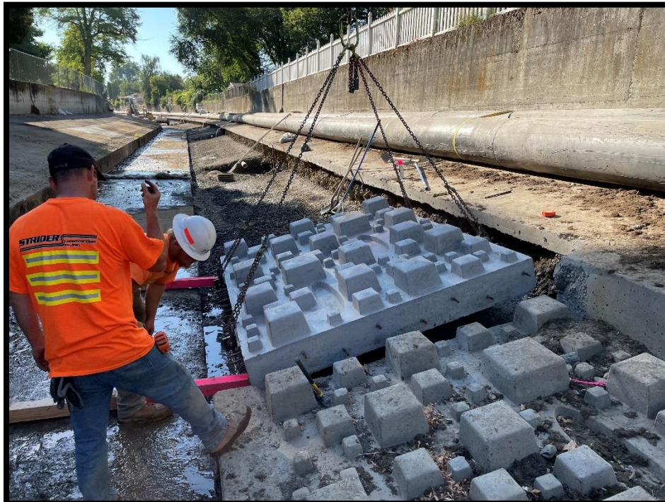
Figure 26: Panels being installed using non-BPA funding in through the State of Washington.
