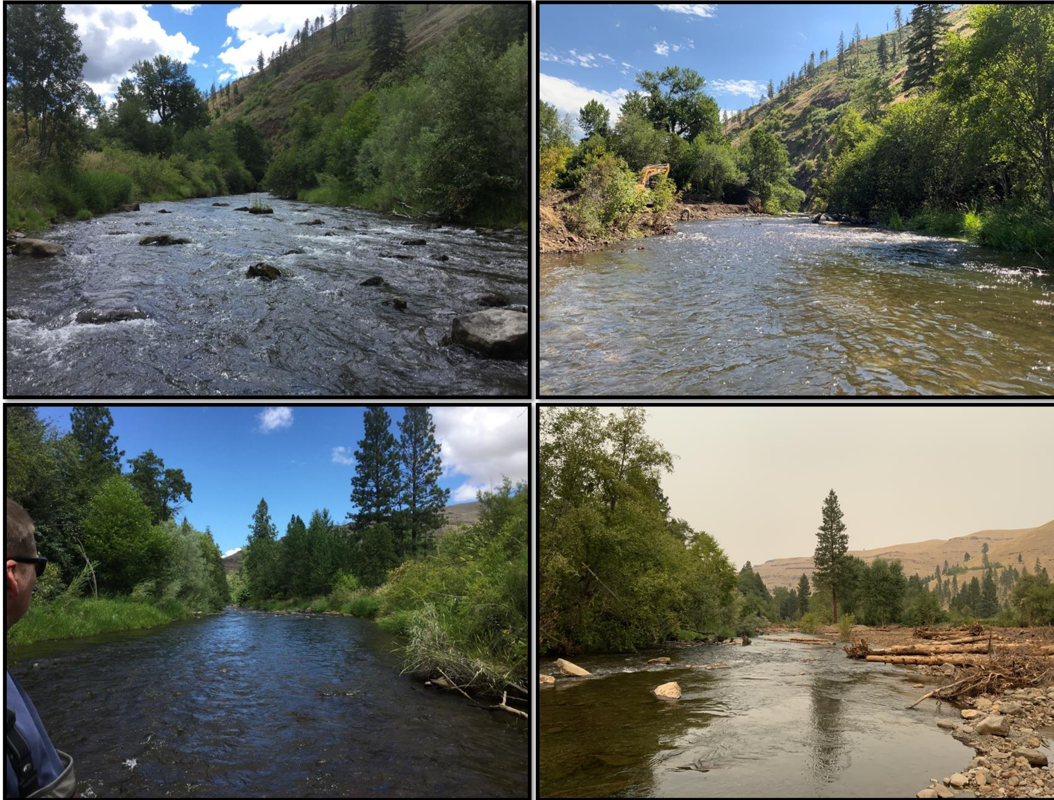
Figure 13-14: Project area 13 channel reached impacted by levee and rip-rap removal pre-project (left upper/lower) and post project as-built 2022. The upper photo set shows the upper leveed section with channel fill placed to elevate water surface to activate low-lying floodplain and side channels.
