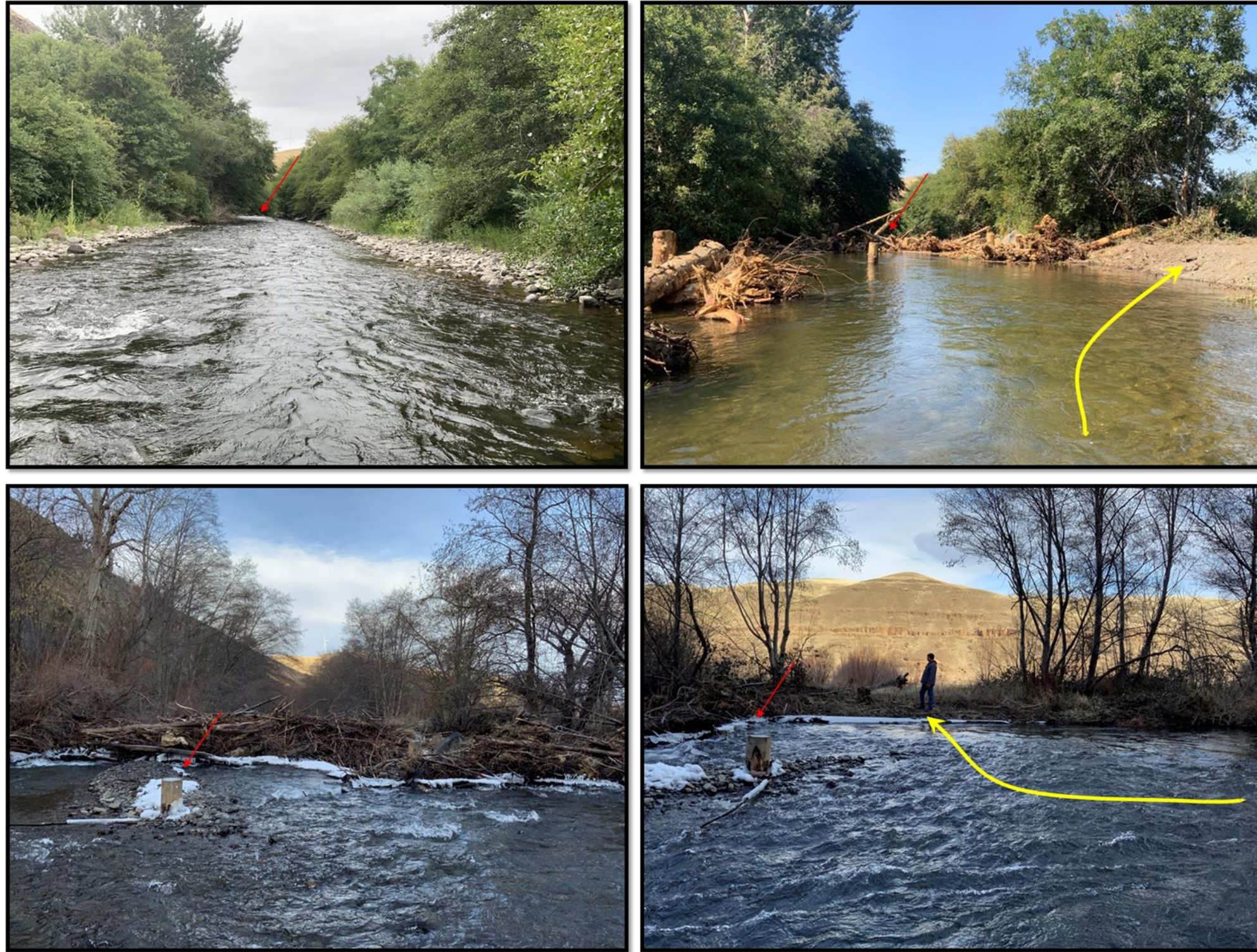
Figure 26-13: Project photo point for channel spanning a structure designed to aggrade the river channel and increase floodplain connectivity, pre-project (upper left) as-built (upper right) and following two high flow events (lower left). The red arrow indicated a reference point pile placed during construction as a test pile and left in position for reference. During the high flow event in December 2022 (Figure 3) channel spanning structures captured significant gravel bed material resulting in an over bank event at less than the 2 yr flow interval indicated by the yellow arrow. Note: The pile when placed was measured to make future observation on bed elevation, which at as-built was measured to emerge 1.4 m out of the stream bed with 0.82 m of it sticking out of the water (upper right). Following two relatively low season low event the bed elevation has aggraded (~1 m) above the original water height with only 0.4 m above the river bed.
