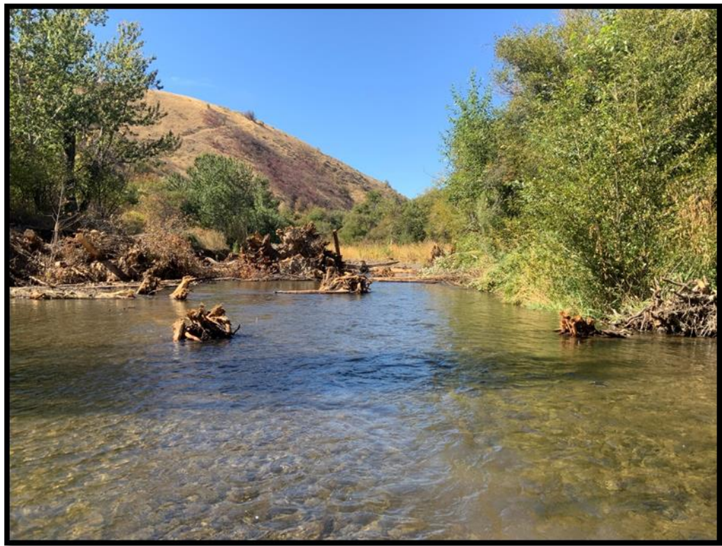
Figure 27/28.1-2: PA28.1 Pre/post Photo Point 2021 illustrating a channel fill reach where thalweg elevation was increased, with LWD secured within the bed matrix.
